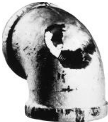
Impingement failure of an elbow that was part of a steam condensate line
