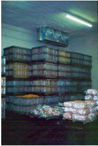
Fig. View of room cooling
